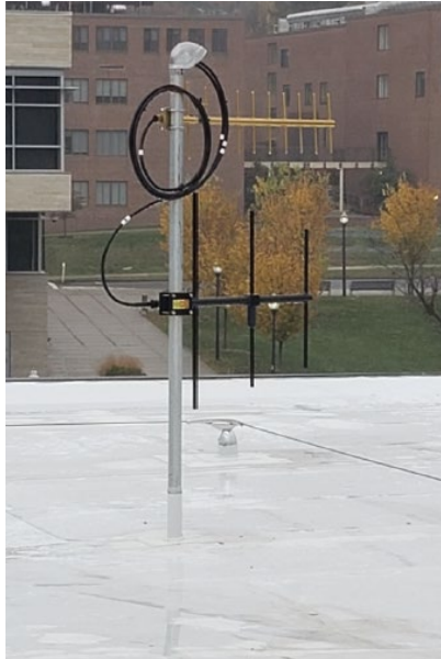
Yagi antenna with roof penetration
