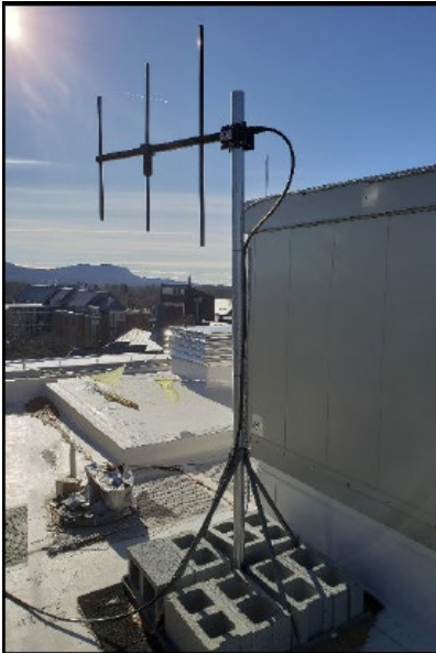
Yagi antenna with non-penetrating roof mount
