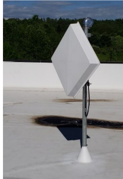
Panel antenna with roof penetration
