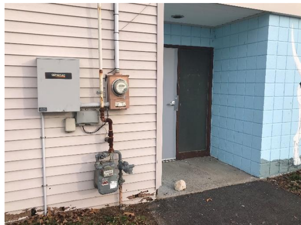
Photo 13-Gas & Electric Meter Location
