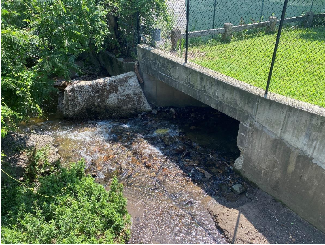
Figure 45: Obstruction at Culvert Outfall
