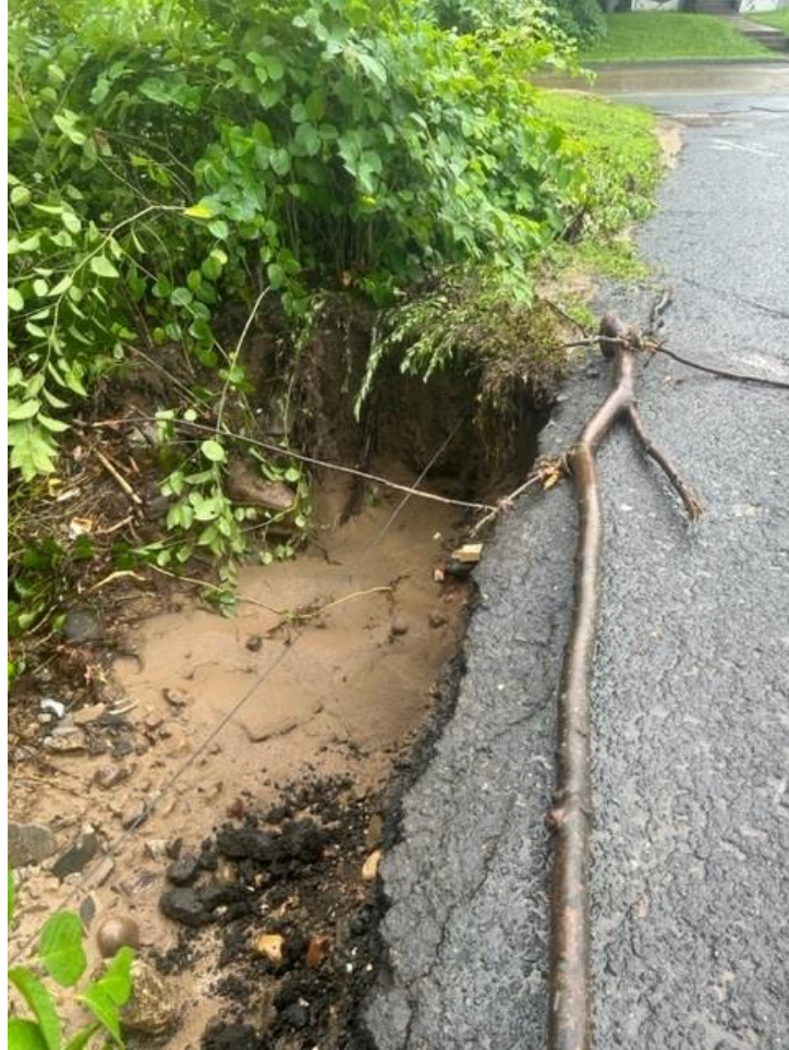
Figure 54: Damaged Driveway on Private Property
