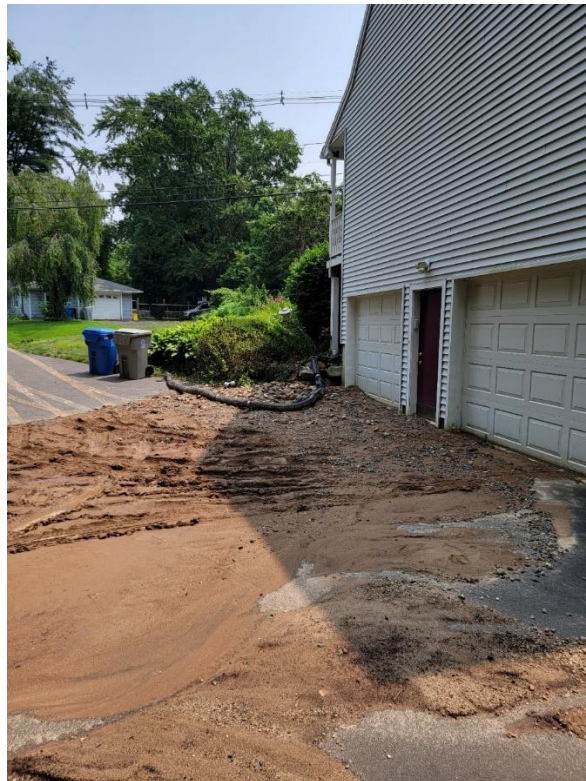
Figure 41: Deposits of Eroded Material
