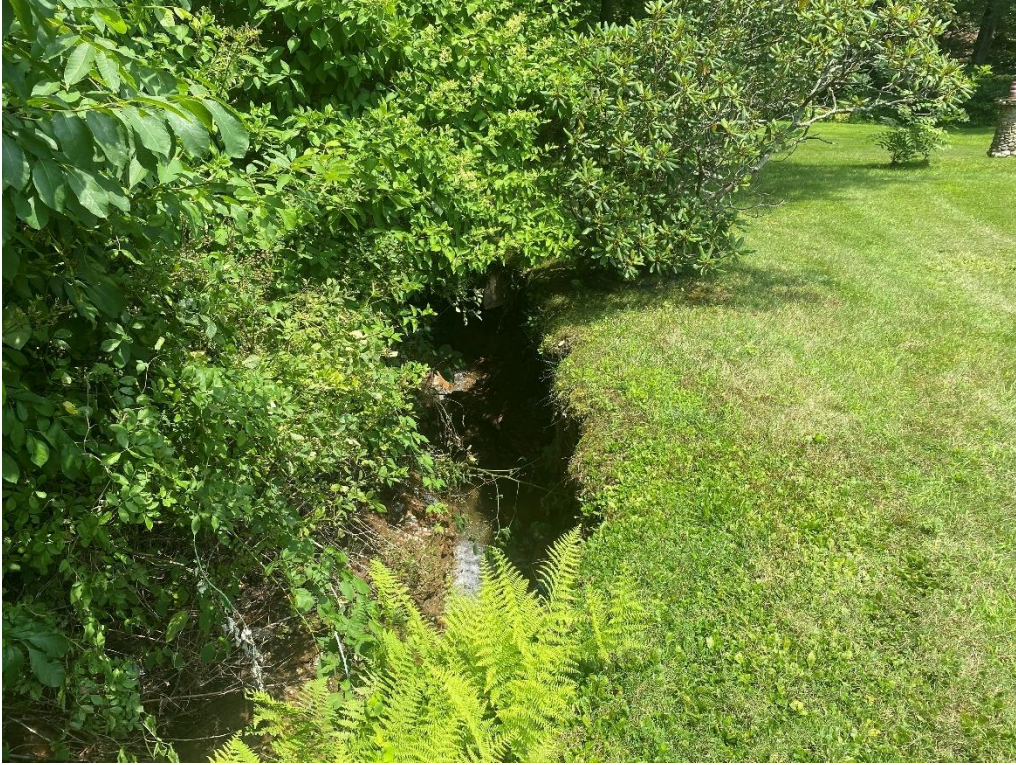
Figure 33: Erosion at Invert of Channel
