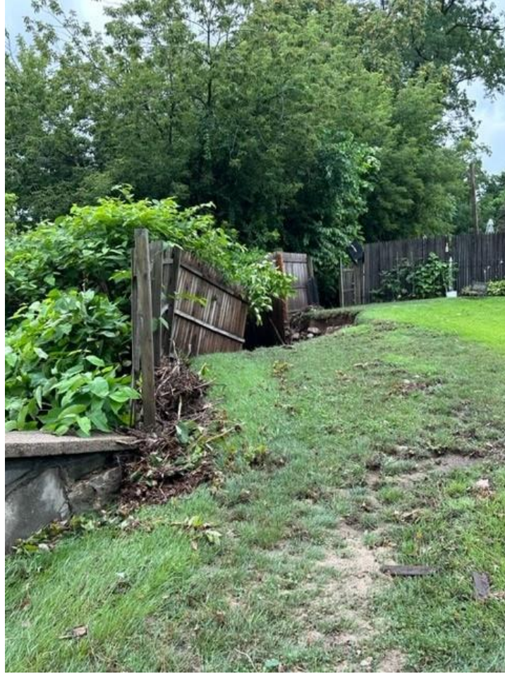
Figure 55: 316 Divinity Street Property Damage
