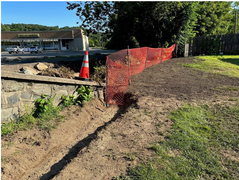
Figure 57: 316 Divinity Street Property Damage
