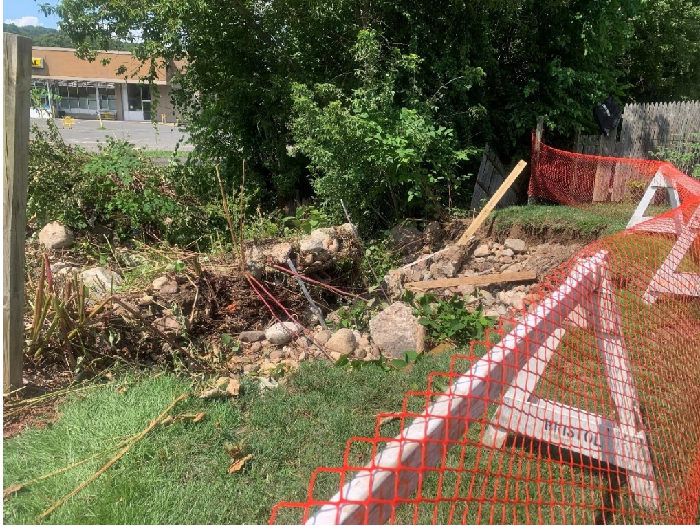
Figure 56: 316 Divinity Street Property Damage
