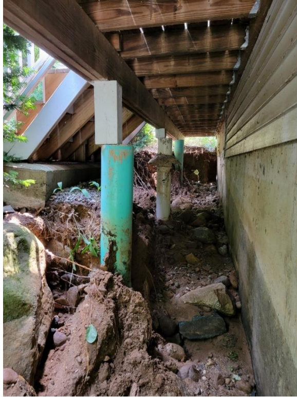
Figure 40: Erosion of Material Caused by Stormwater
