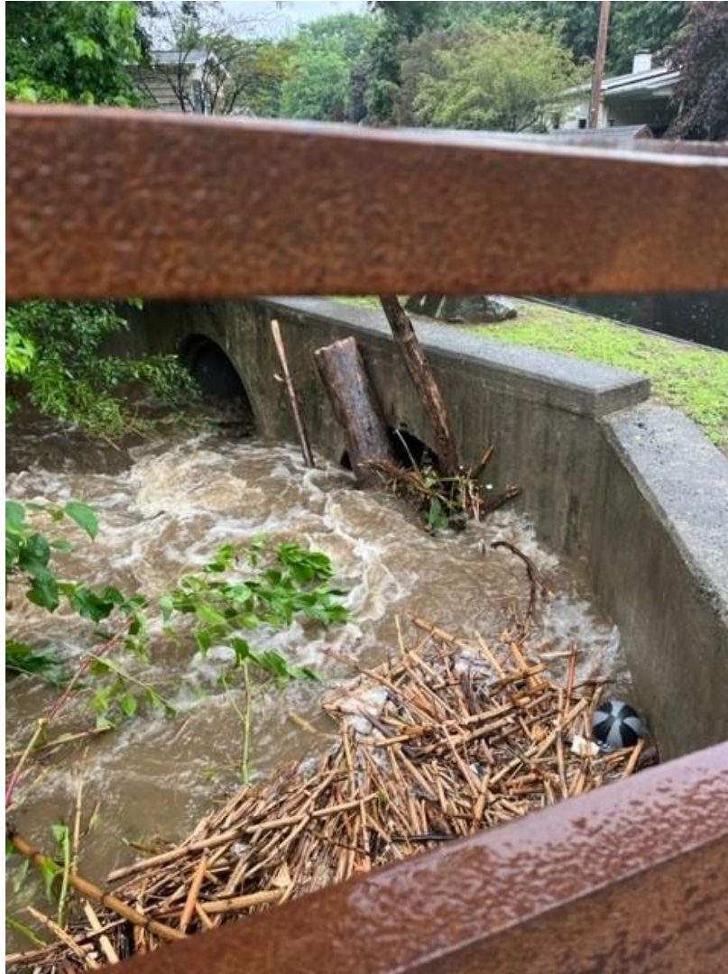
Figure 44: Debris Blocking Flows at Culvert
