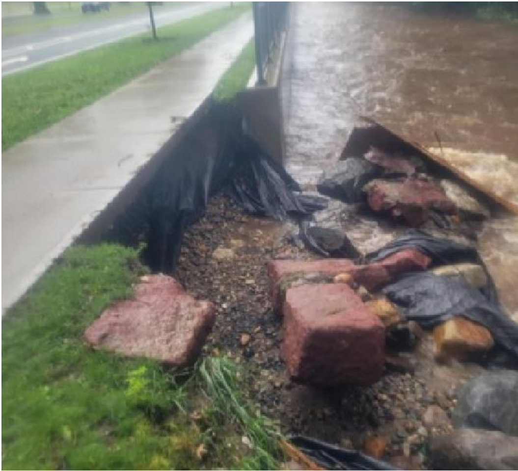
Figure 47: Collapse of Existing Dry Stack Stone Wall
