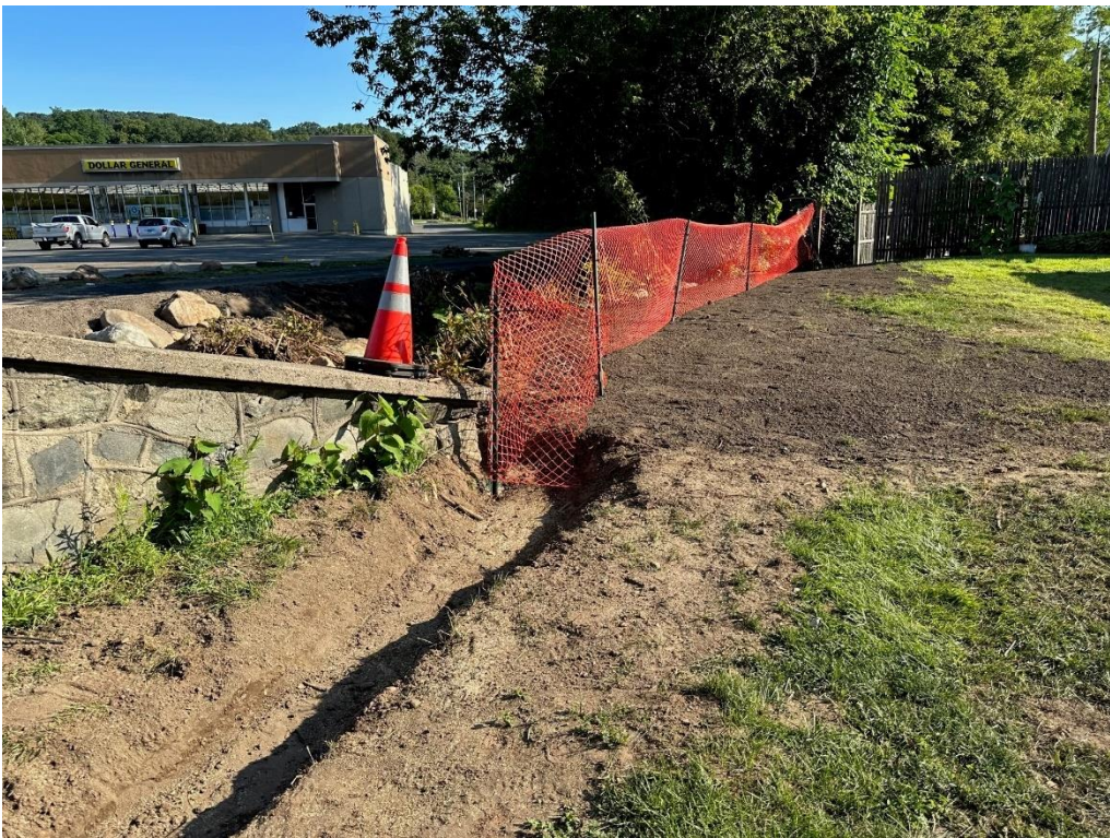
Figure 66: 316 Divinity Street Property Damage
