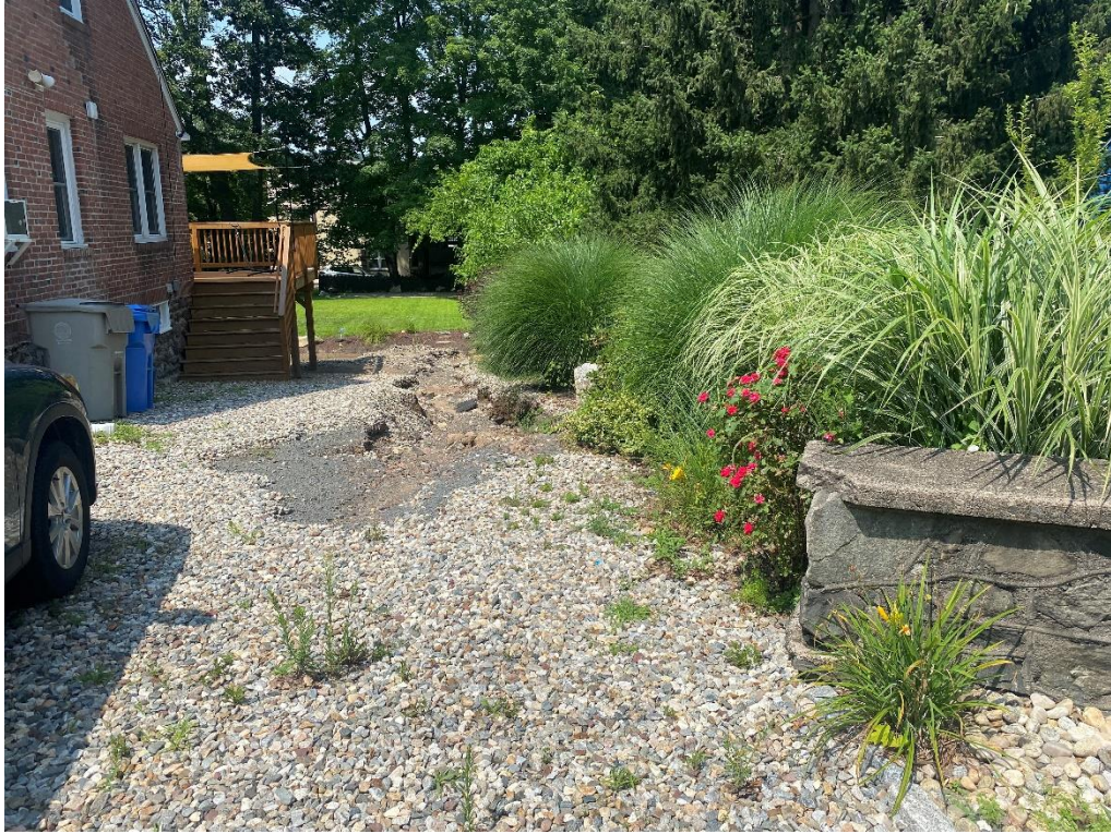
Figure 24: Erosion of Unpaved Driveway
