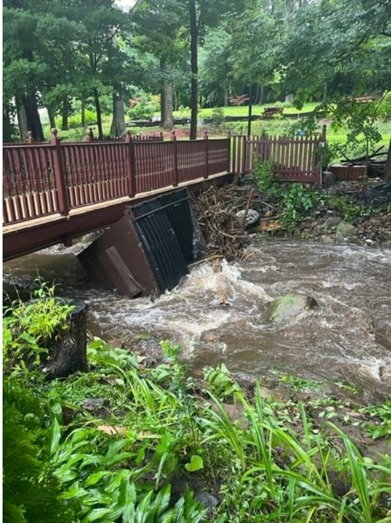
Figure 71: Dumpster Obstructing Flows
