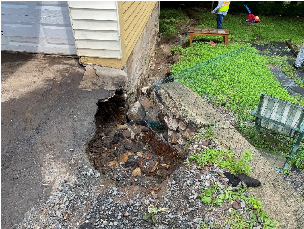
Figure 18: Erosion Behind Existing Retaining Wall
