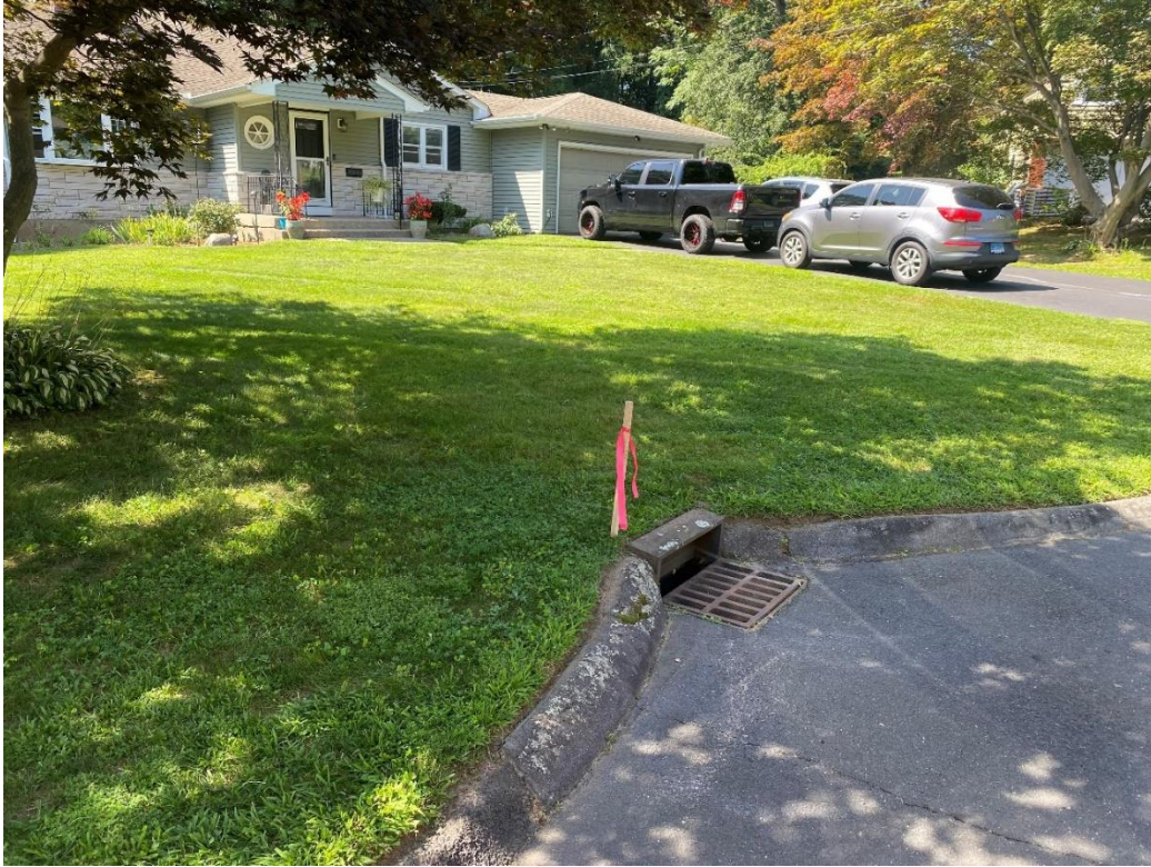
Figure 10: Substandard Catch Basin To be Replaced
