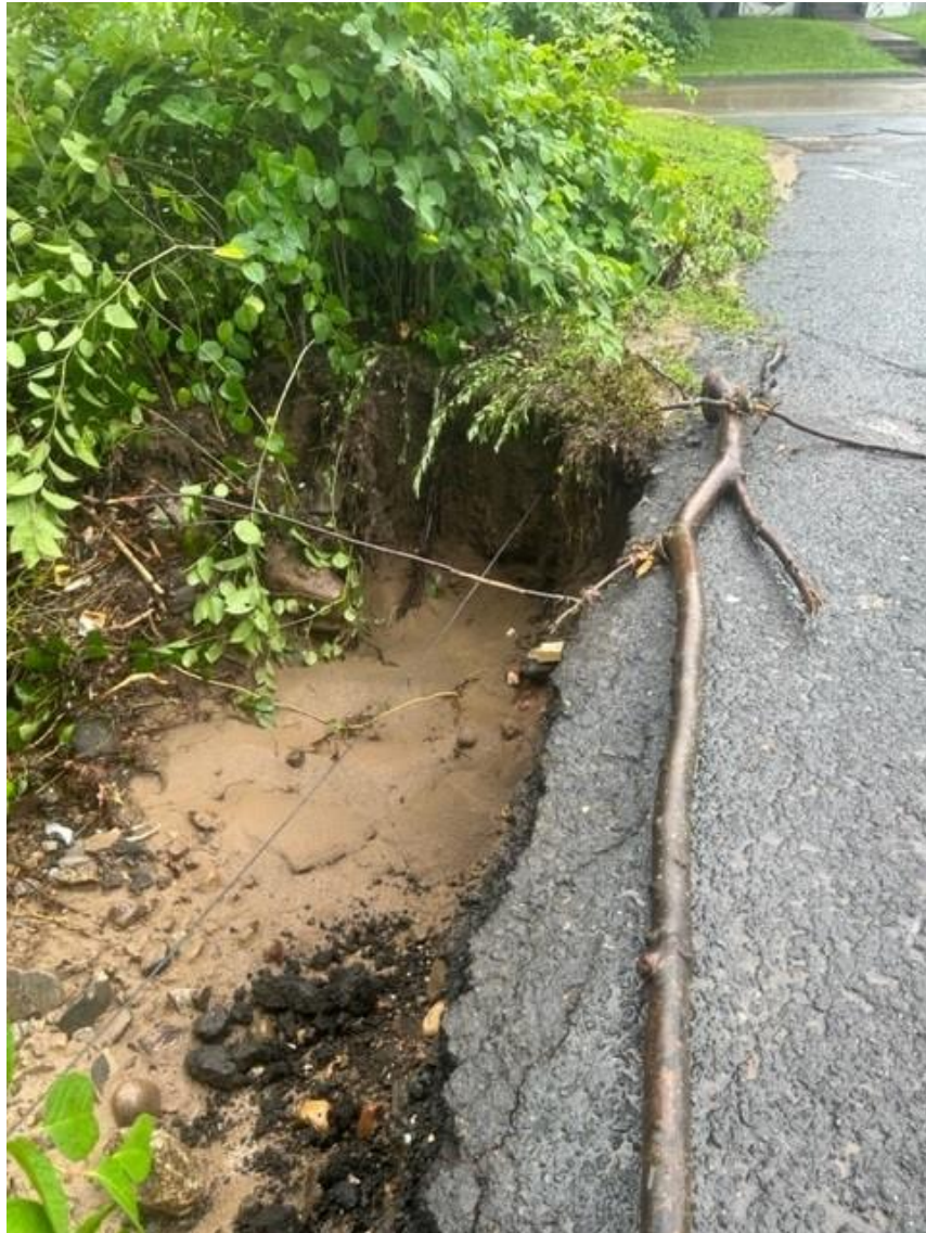
Figure 63: Damaged Driveway on Private Property
