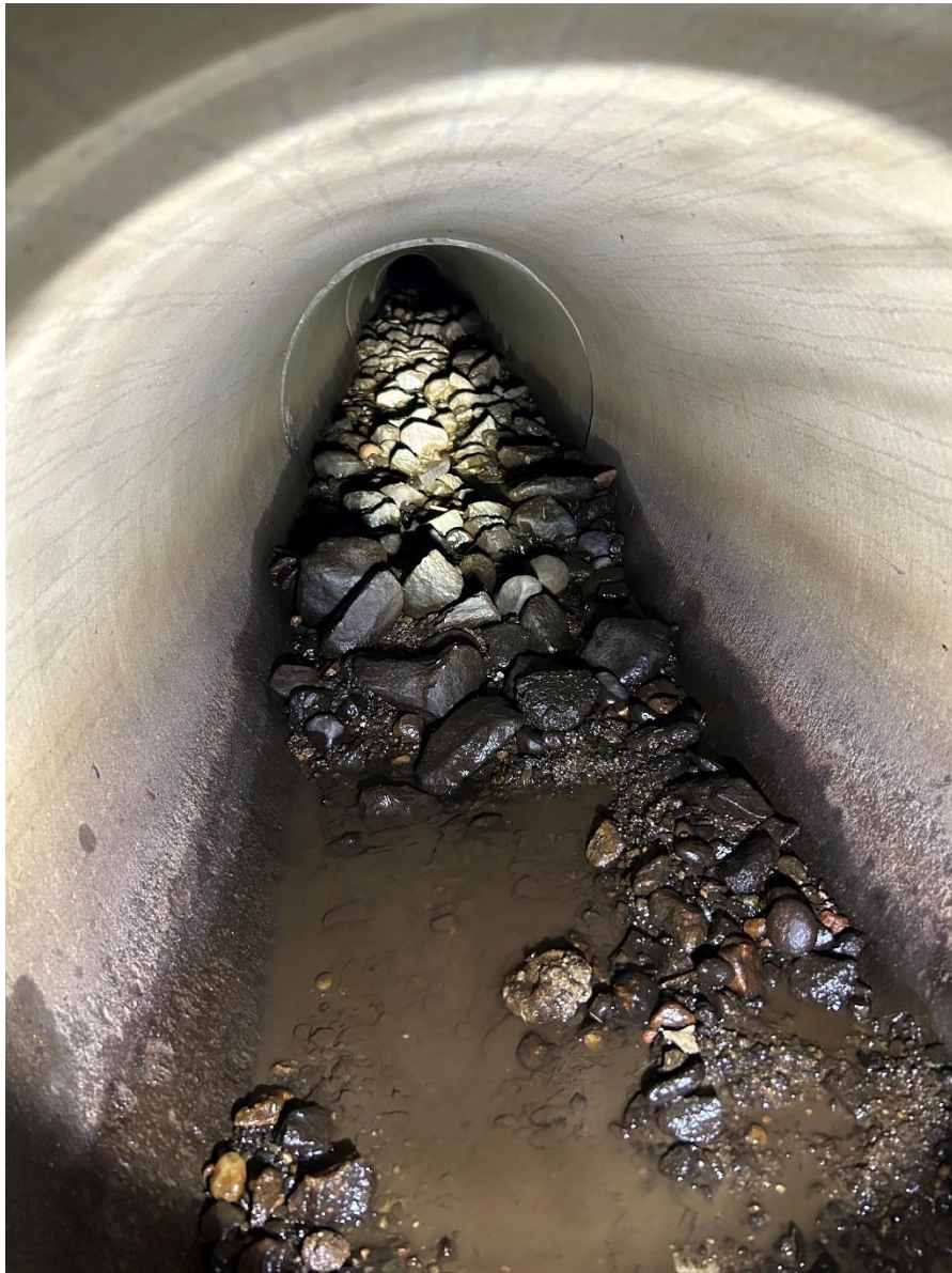
Figure 36: Obstruction Within Existing Pipe
