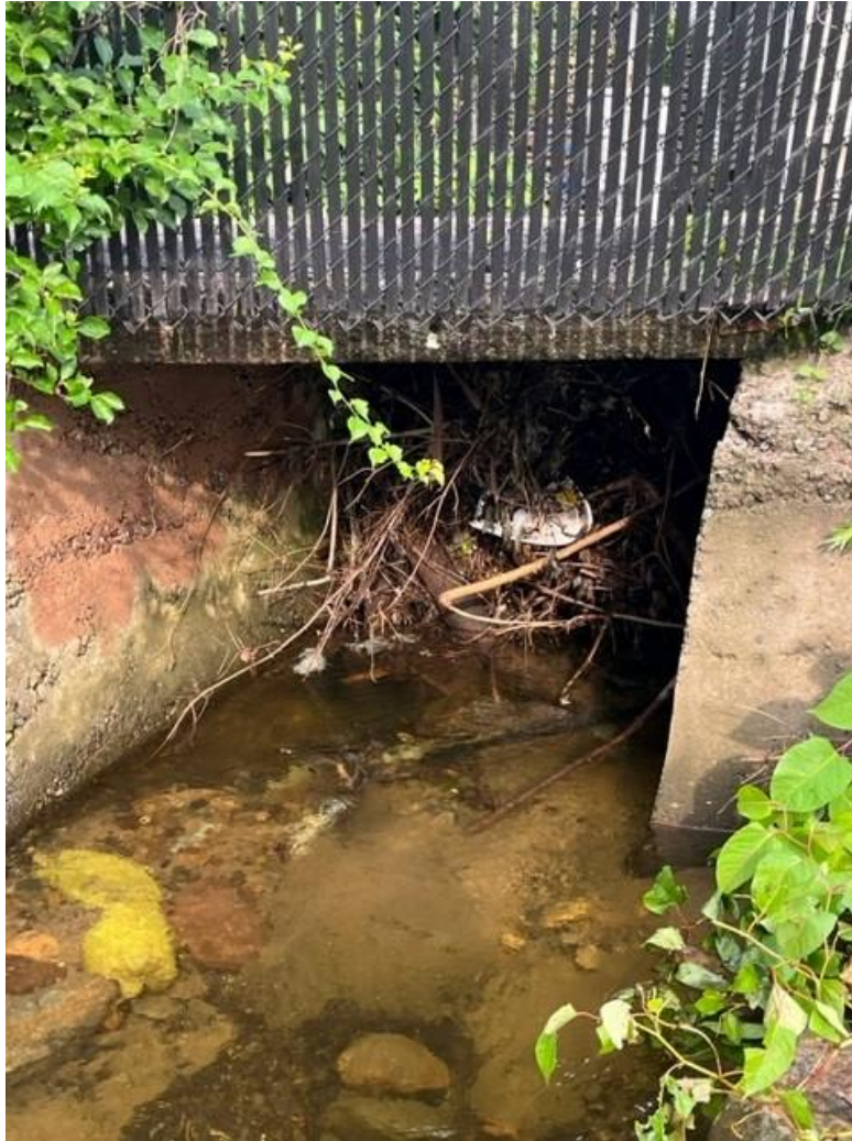
Figure 70: Buildup of Debris Within Private Culvert
