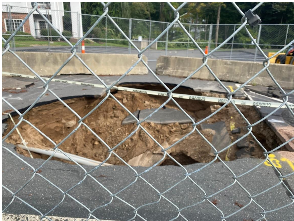
Figure 15: Sinkhole Located Overtop of Existing Culvert
