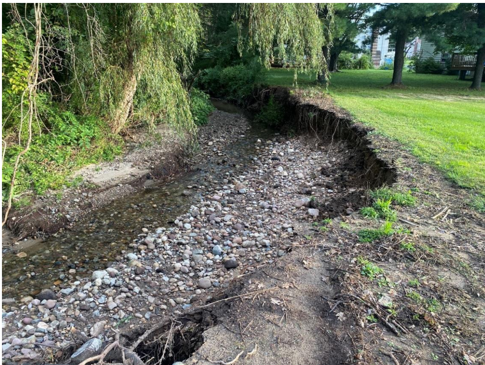
Figure 7: Current Condition of East Bank
