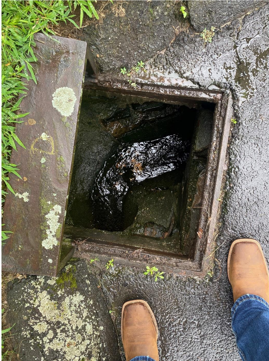
Figure 11: Substandard Catch Basin To Be Replaced
