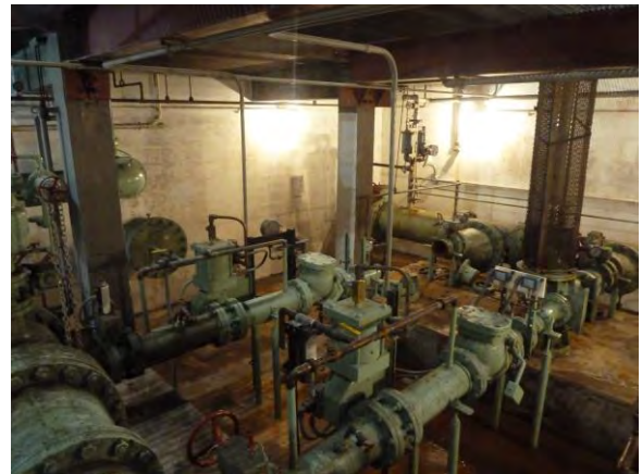
Lower Wellfield Pumping Station lower level
