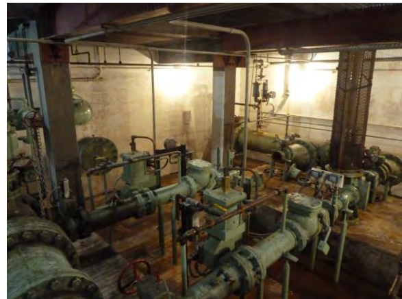
Lower Wellfield Pumping Station lower level
