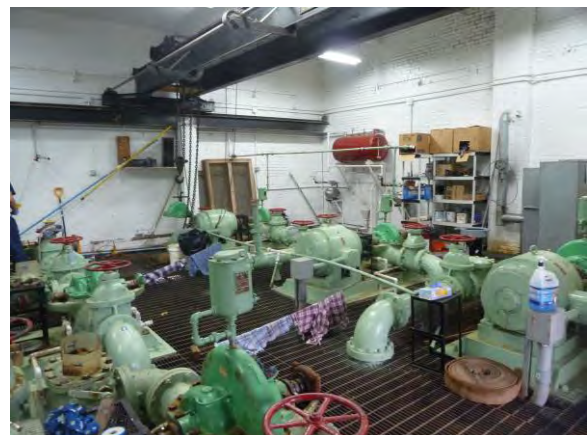
Pond Pumping Station internal pump and piping
