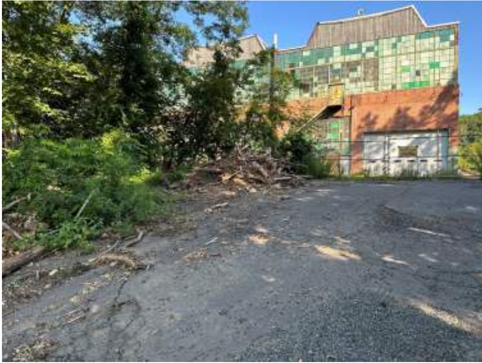
Figure 59: Debris Removed from Channel
