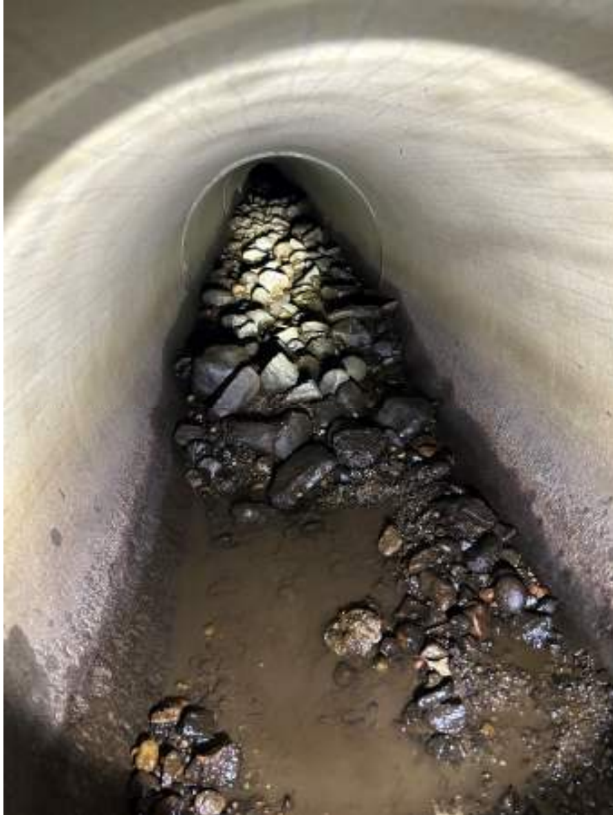
Figure 35: Obstruction Within Existing Pipe
