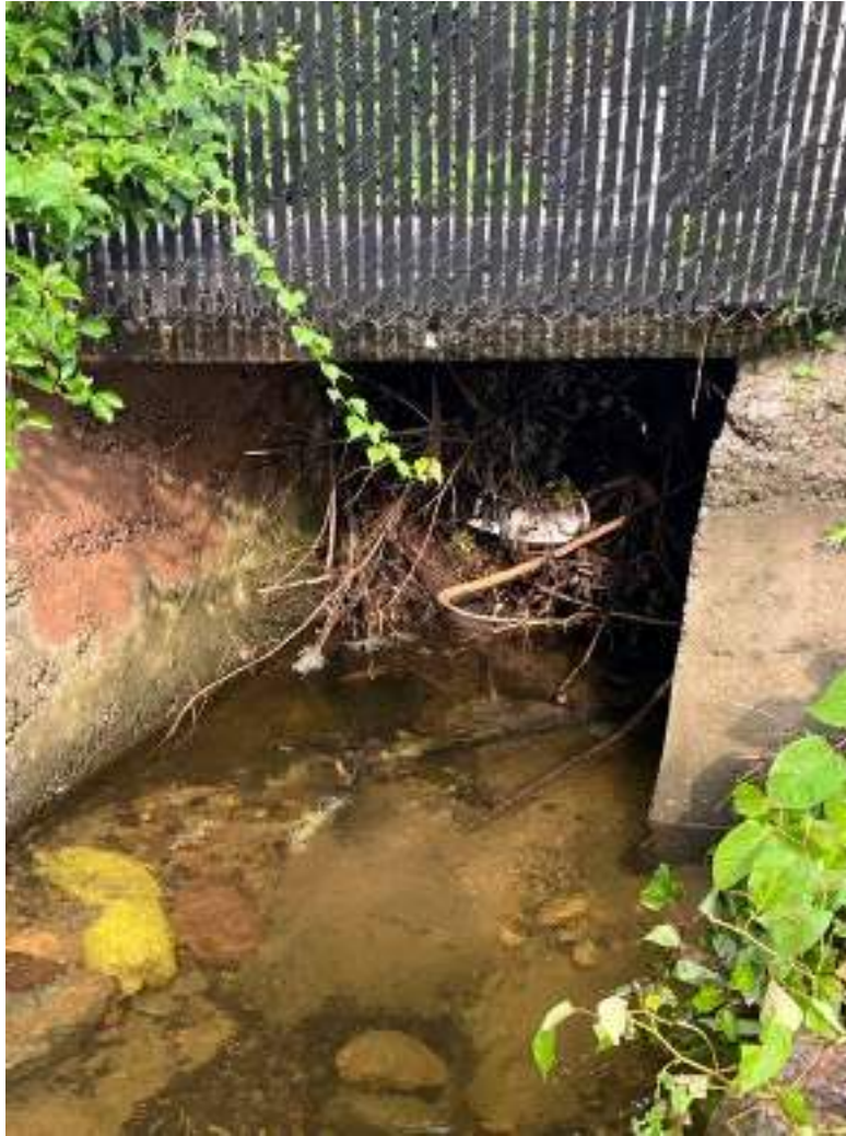
Figure 69: Buildup of Debris Within Private Culvert
