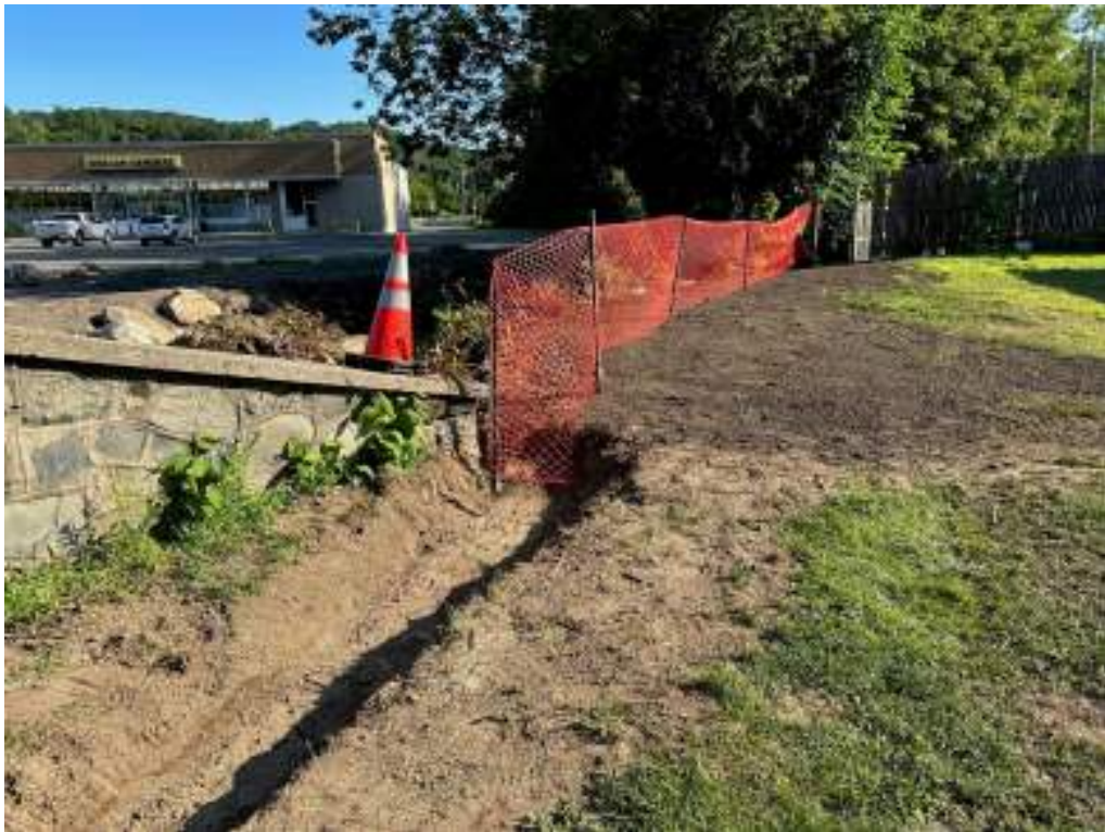
Figure 65: 316 Divinity Street Property Damage
