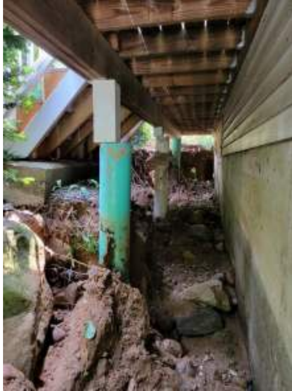
Figure 48: Erosion of Material Caused by Stormwater
