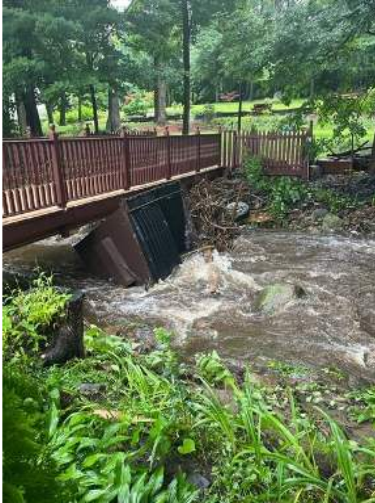
Figure 70: Dumpster Obstructing Flows
