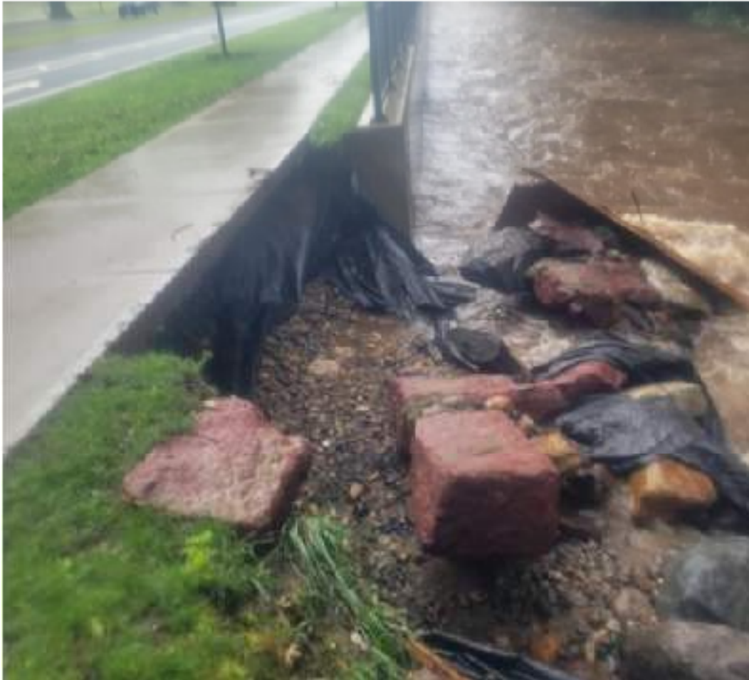
Figure 55: Collapse of Existing Dry Stack Stone Wall
