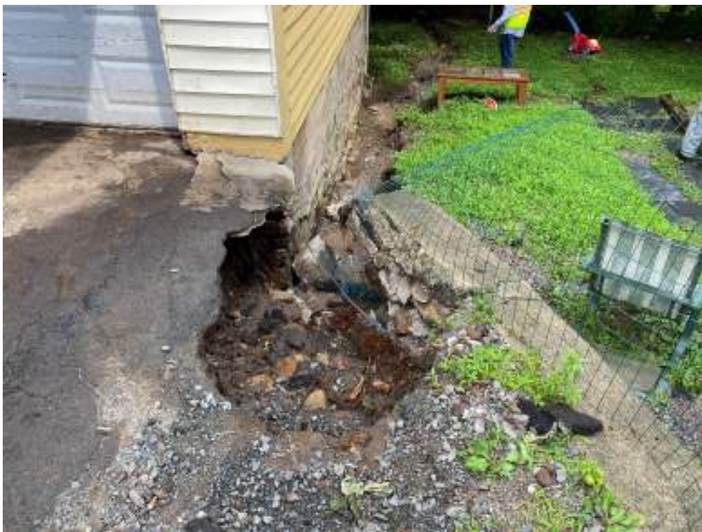
Figure 17: Erosion Behind Existing Retaining Wall
