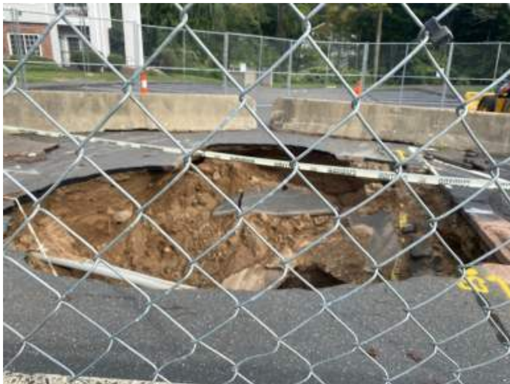
Figure 14: Sinkhole Located Overtop of Existing Culvert
