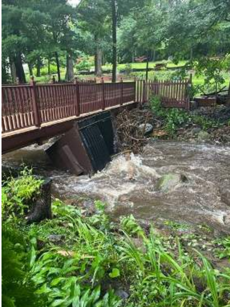
Figure 70: Dumpster Obstructing Flows
