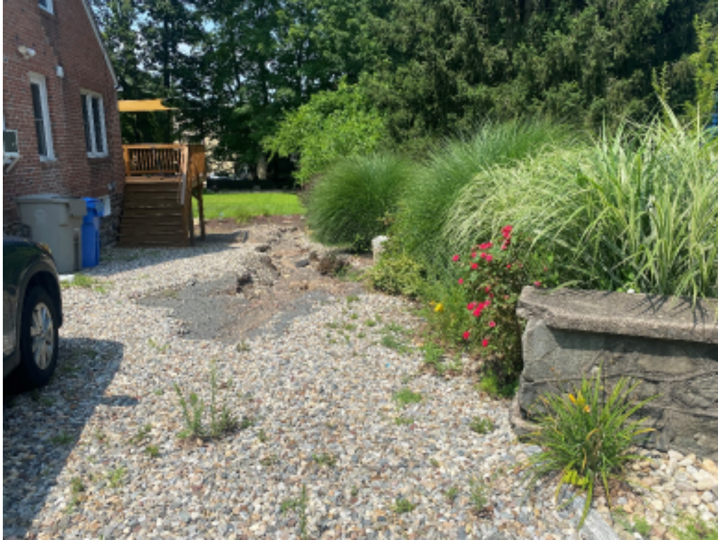
Figure 23: Erosion of Unpaved Driveway
