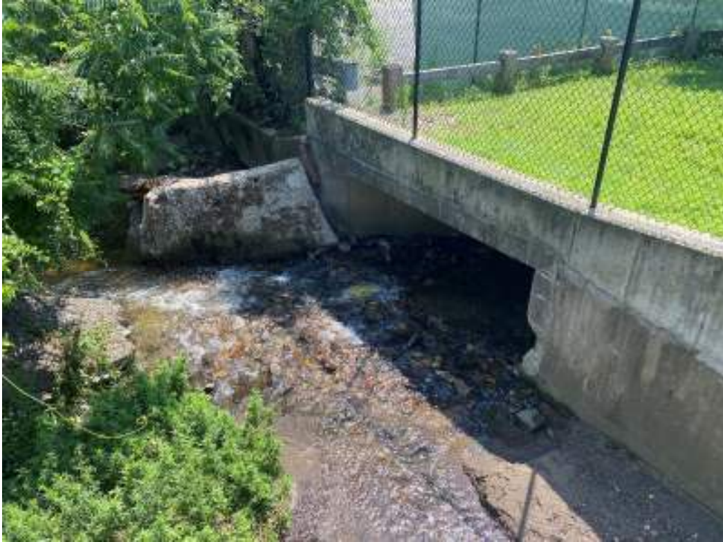
Figure 53: Obstruction at Culvert Outfall
