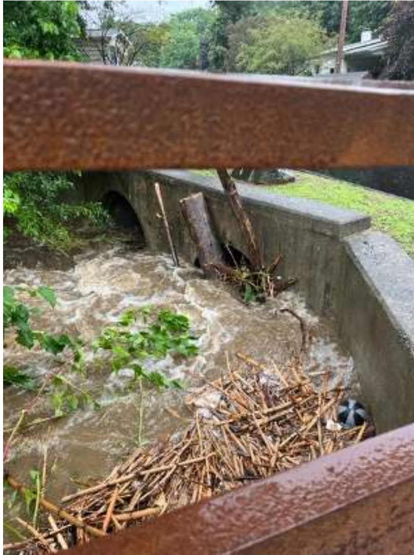
Figure 52: Debris Blocking Flows at Culvert
