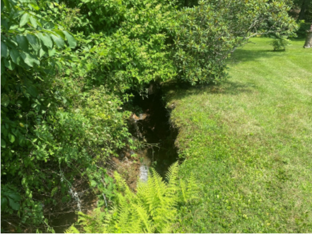
Figure 40: Erosion at Invert of Channel
