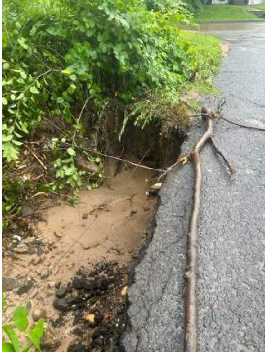
Figure 62: Damaged Driveway on Private Property
