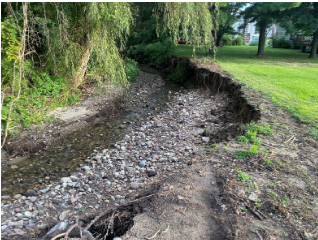
Figure 7: Current Condition of East Bank
