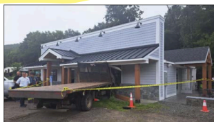
Jimmy Driscoll, owner of Jimmy's On The River. The damage to Jimmy's On The River after it was struck by a vehicle for the second time in two years.
