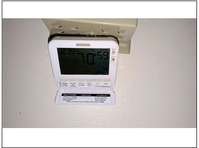
8. Wall mounted thermostat controlling packaged rooftop unit
