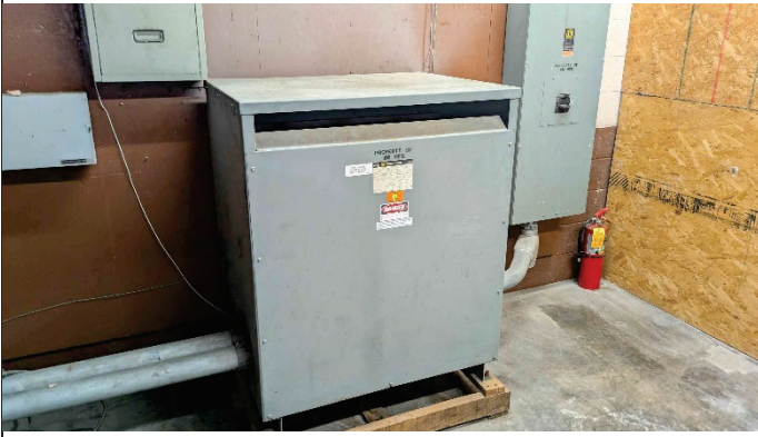
13. 300 KVA Step up transformer serving bus bar in area previously utilized as a production floor
