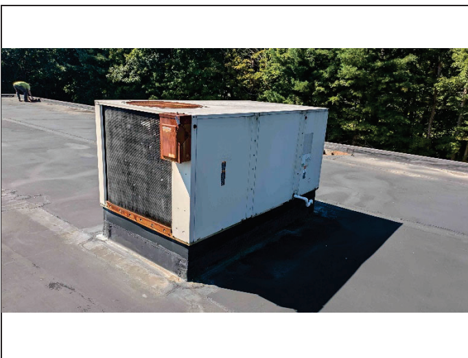
5. 7.5 Ton packaged rooftop unit serving production area
