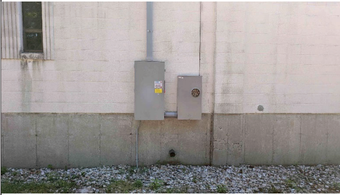
15. 400A, 480-V, 3-phase Service disconnect and utility meter
