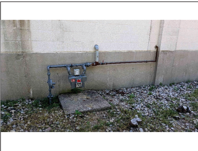
3. Property natural gas utility meter
