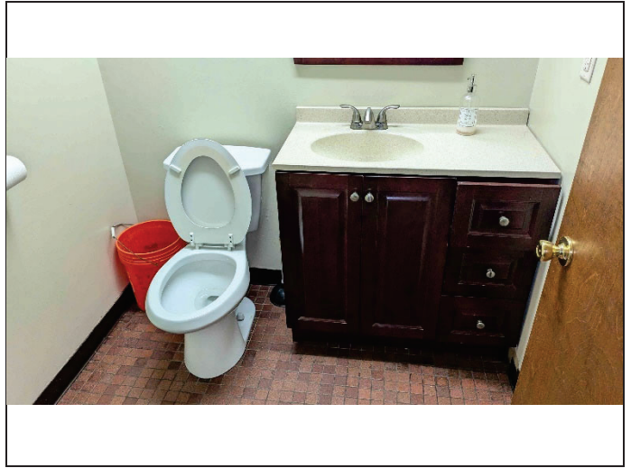
2. Office space plumbing fixtures
