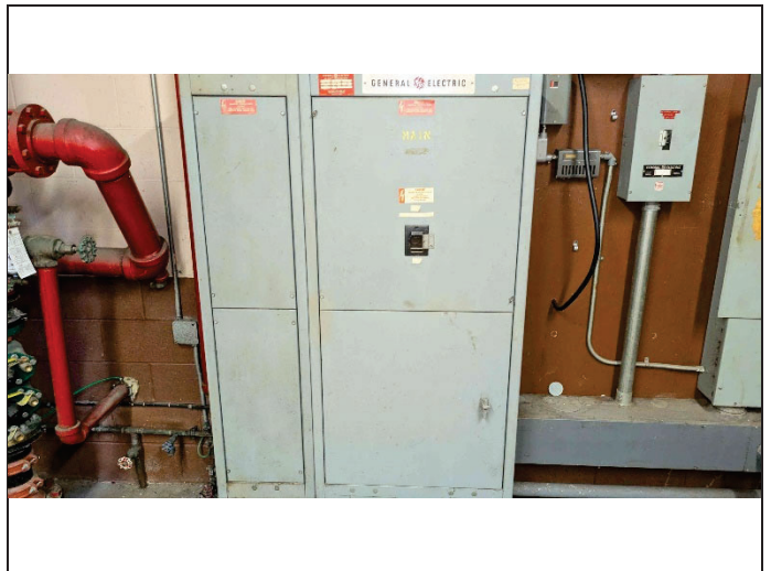
10. 800A, 208-Volt, 3-phase electrical service switch
