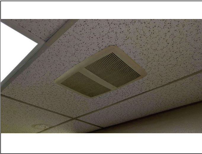
7. Restroom ceiling mounted exhaust fan located in office area
