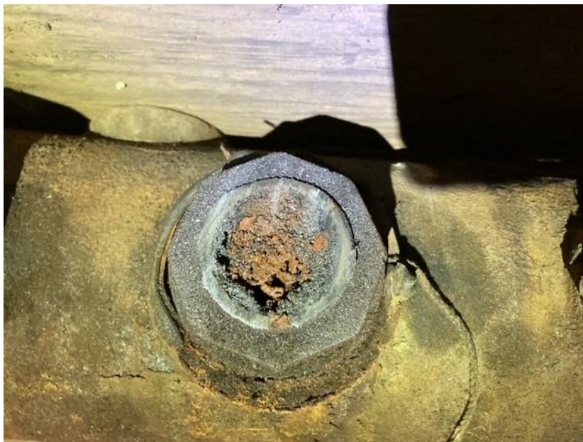
A mud drum nipple that was completely clogged with mineral scaling
