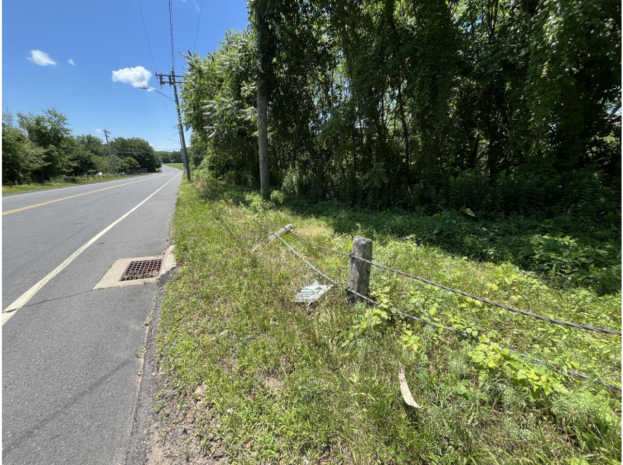
Figure 2: Damaged Timber Post Cable Guiderail
