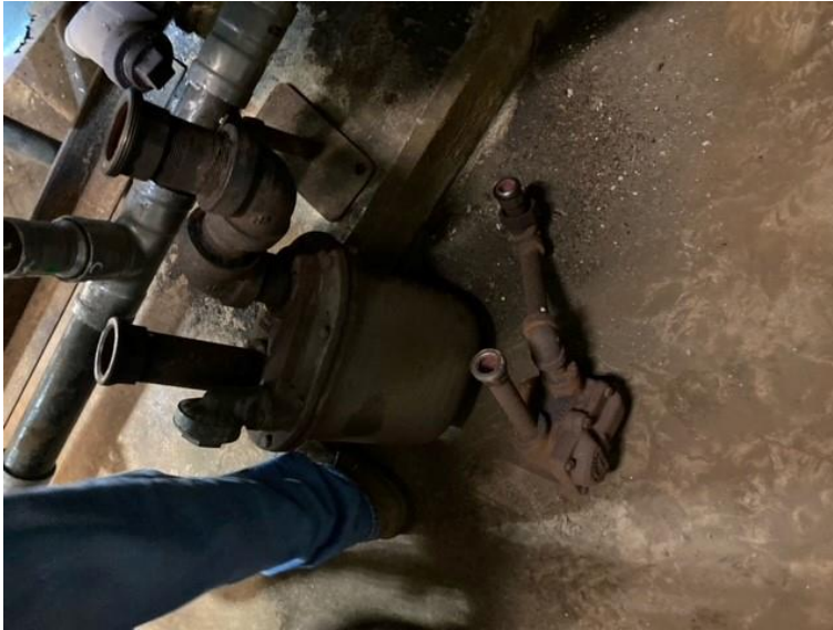
Two condensate tank steam traps that required replacement due to age
