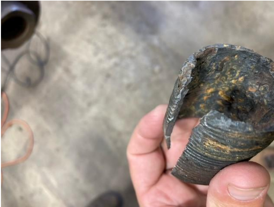
Mud drum nipple that required being cut-out during re-conditioning at Oakland LLC
