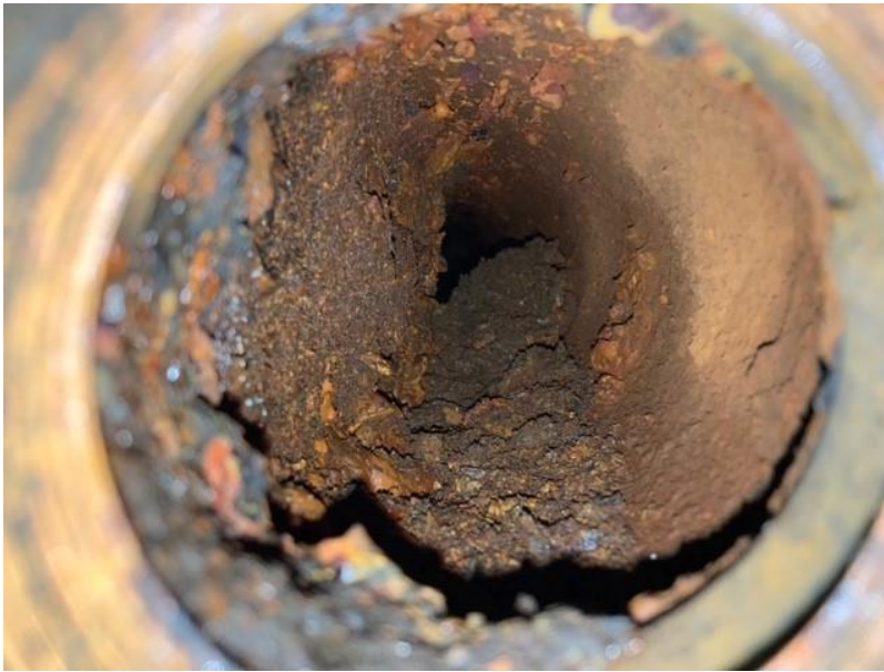
Mud drum exhibiting decades of mineral scaling that was air-chiseled out during re-conditioning.
