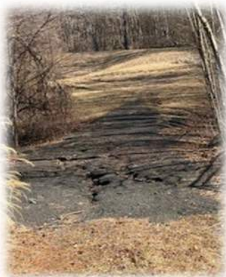
Photo: Erosion at access drive
