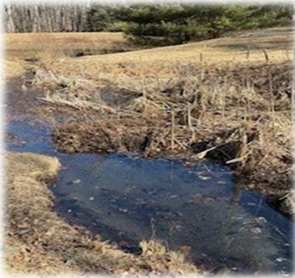
Photo: Sediment and cattails in forebay
