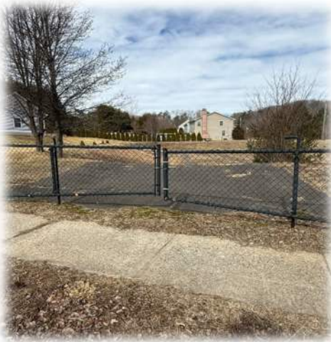
Photo 1: Warner St gate lock missing
