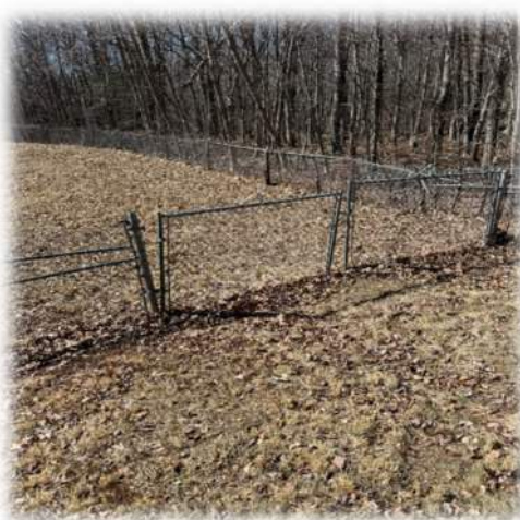
Photo 2: Broken fence gate
