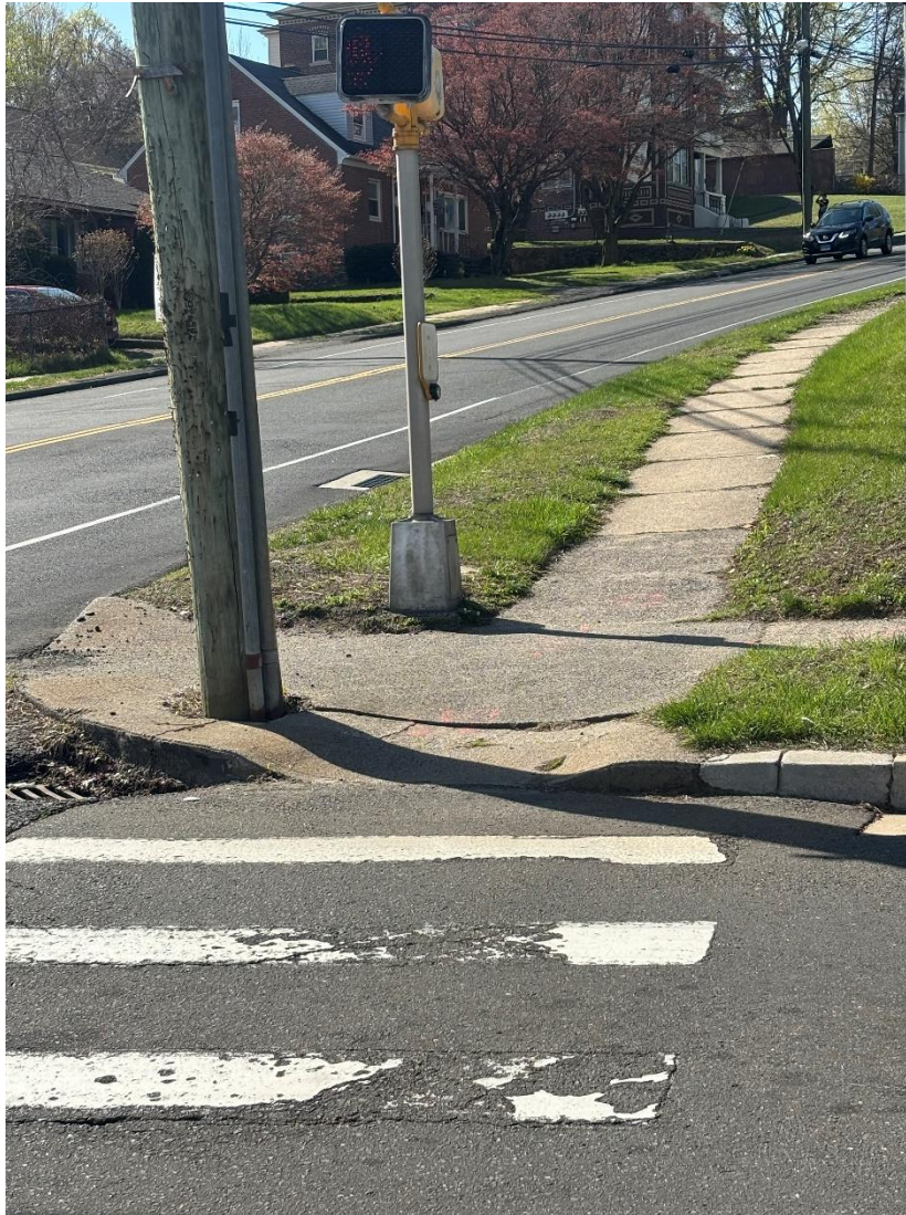
Figure 3: Existing Ramp - Infeasible Under PROWAG / ADA – Intersection @ West St. & South St.
