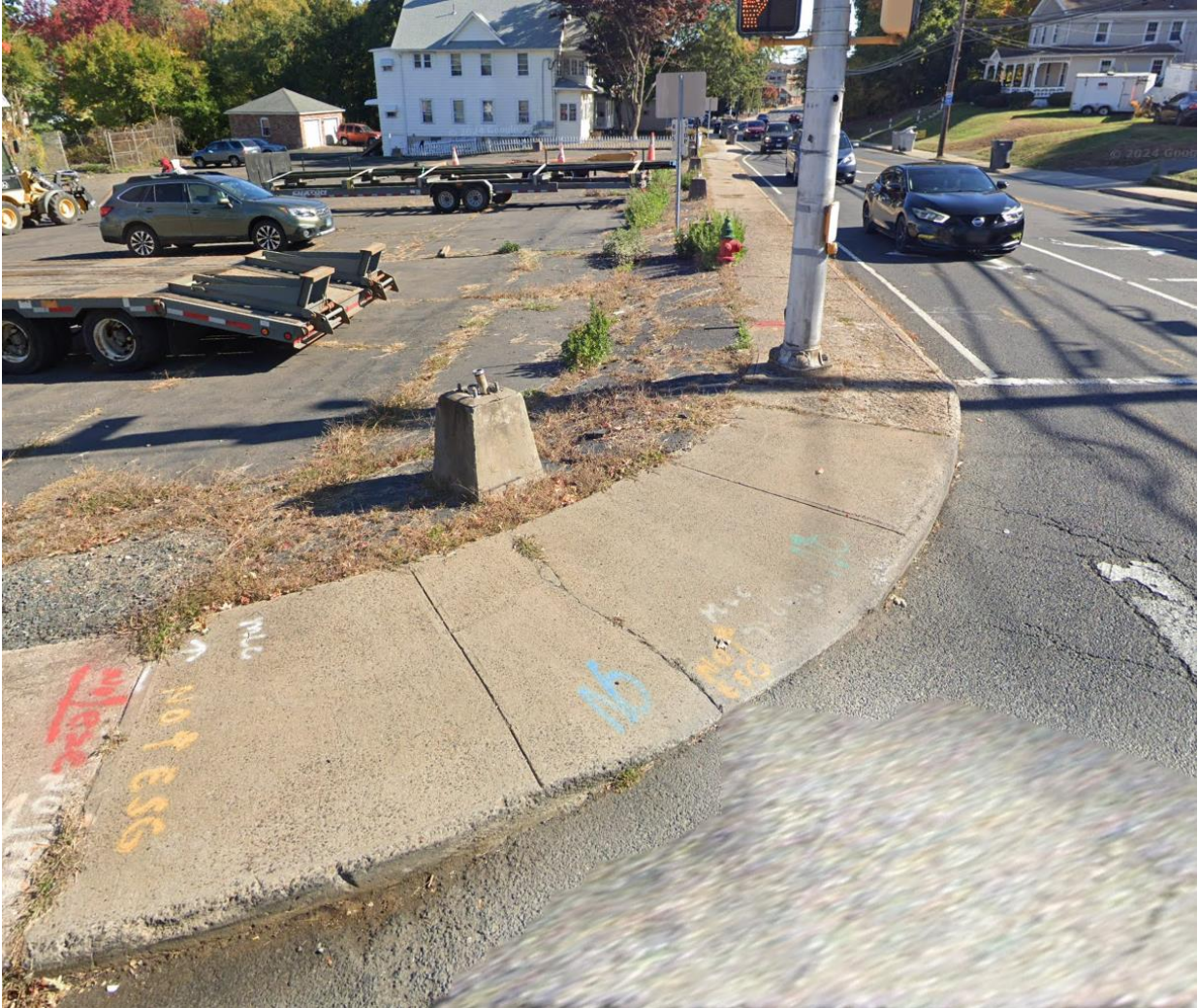
Figure 1: Existing Ramp – Non Compliant
