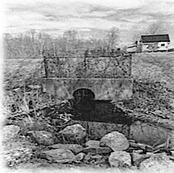
Photo 2: Vegetation covering fence
