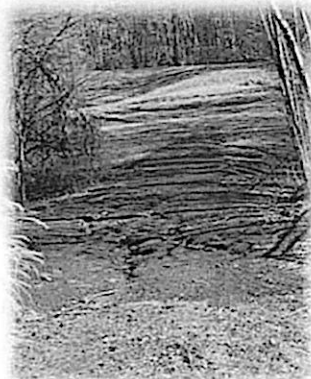
Photo: Erosion at access drive
