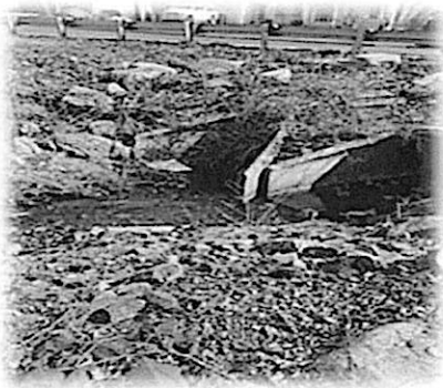
Photo: Flared end outlets
