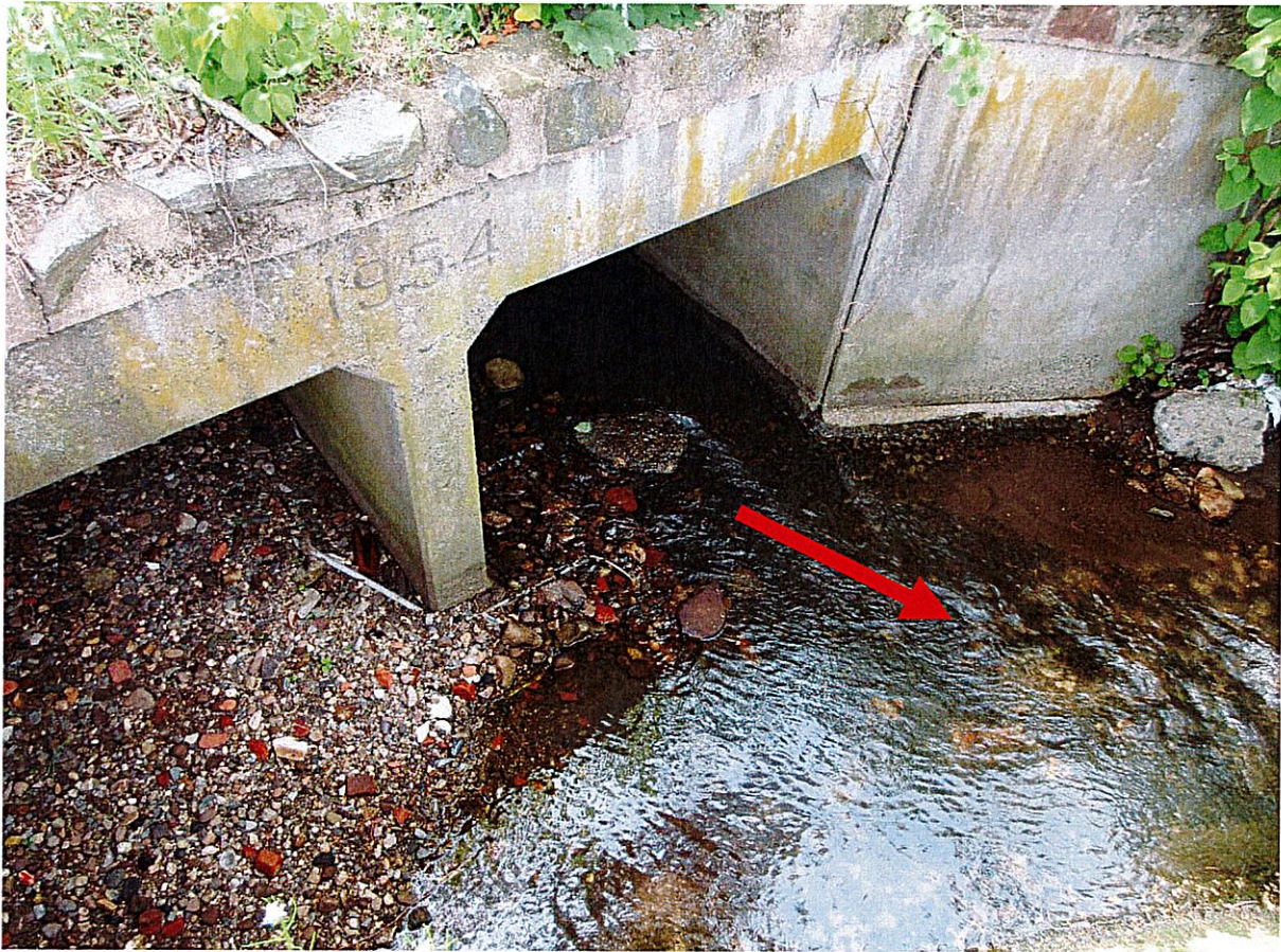
Photo 11b: Park1 (photo taken 05/27/2025 during reconnaissance) Photo depicts the cloudy water observed during the reconnaissance. Red arrow shows flow direction.
