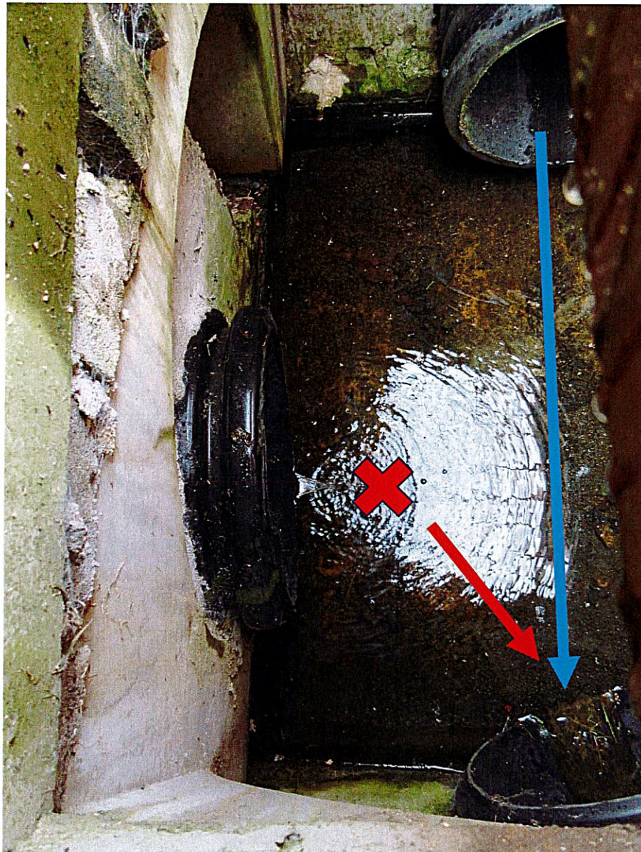
Photo 9: Gridley1 (photo taken 05/28/2025 at approx. 10:10) Outfall located at 221 Gridley St, Bristol, Ct. Red arrows show flow direction from outfall. Blue arrow shows flow- through direction of interconnected storm pipes.
