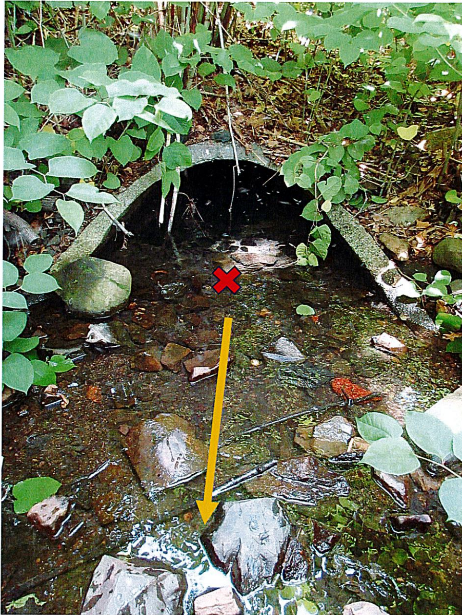
Photo 12: Greene1R (photos taken 05/28/2025 at approx. 11:52) Outlet of an unnamed culverted stream located at the end of 102 Greene St, Bristol, CT. The outflow joins with the discharge from Greene1L approximately 10 feet downstream. Sample point is indicated by a red X. Arrow shows flow direction. See associated photo: 13b : which is labeled to show the confluence between the culverted stream (yellow arrow) and Greene1R stream (blue arrow) as well as directional flow.
