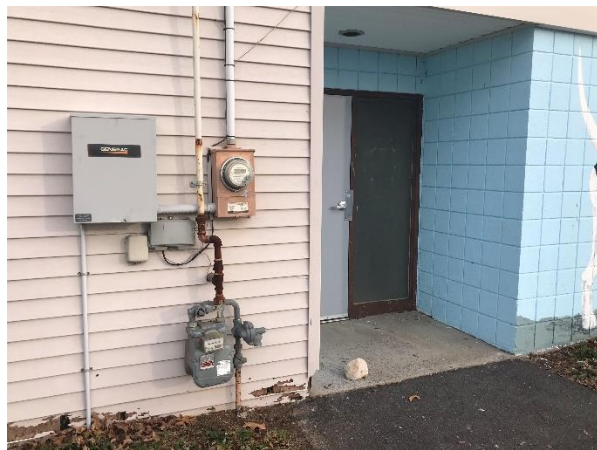
Photo 13-Gas & Electric Meter Location
