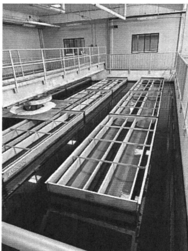
Sedimentation tanks to be retrofitted with new equipment
